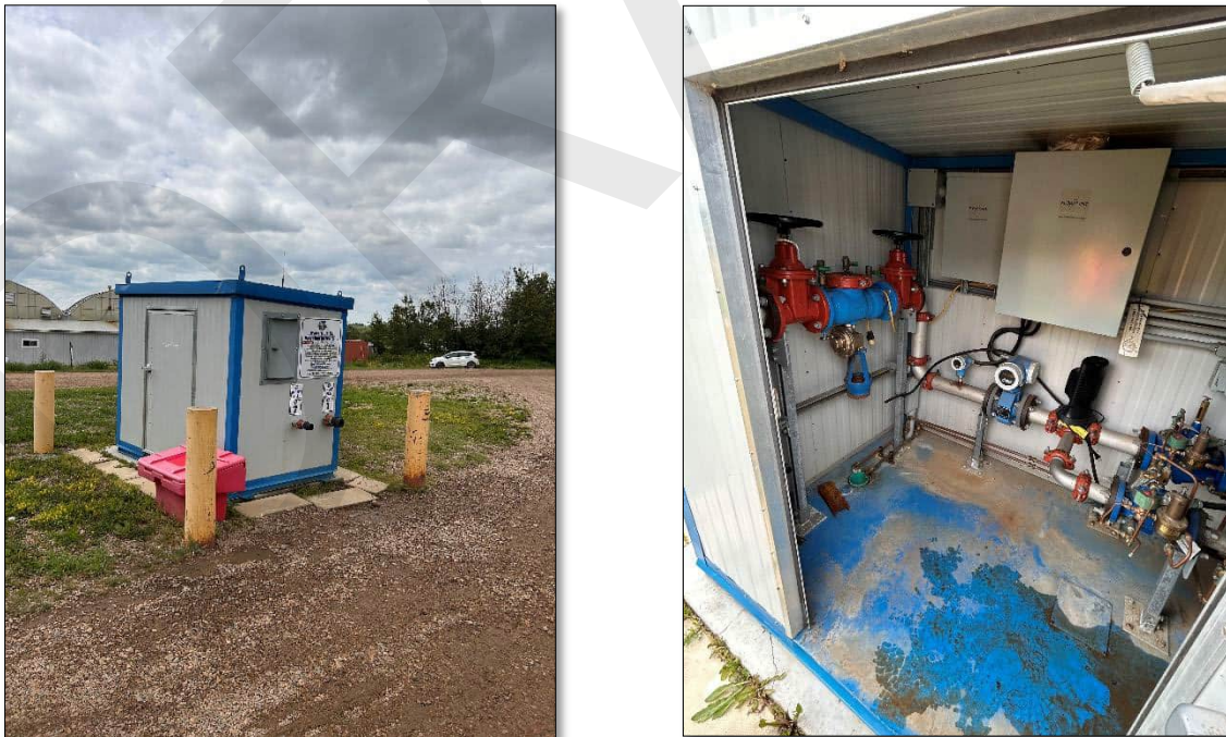
Figure 2.3: Bulk Water Distribution Station
