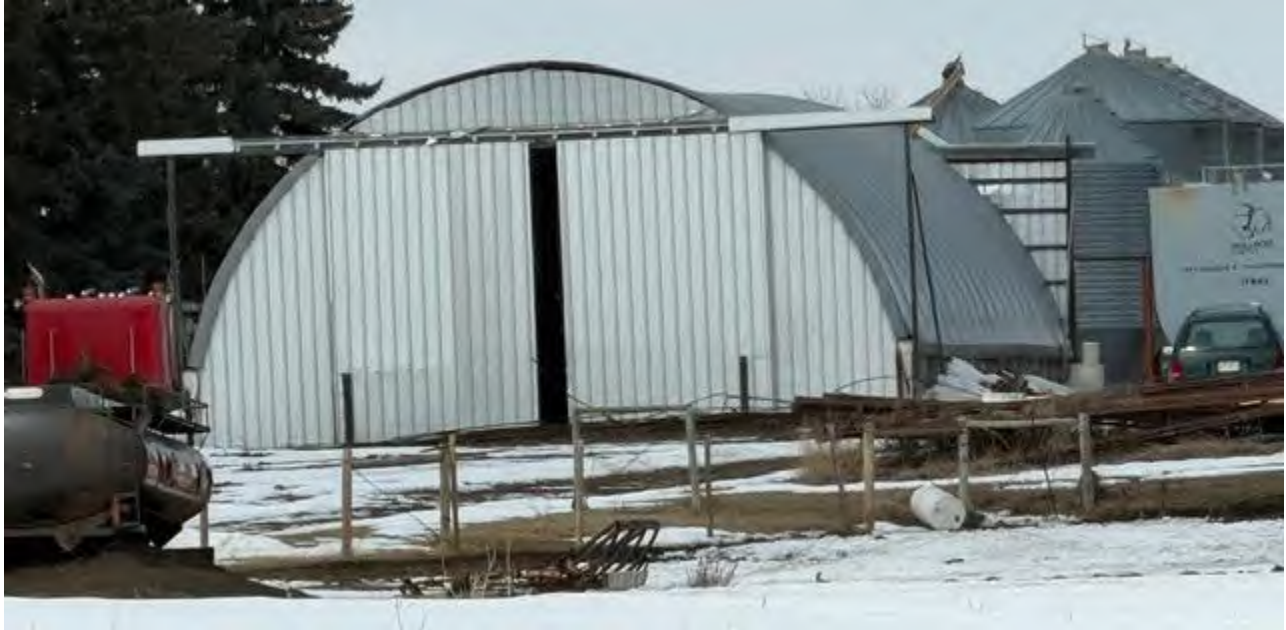
Quonset without permit approval
