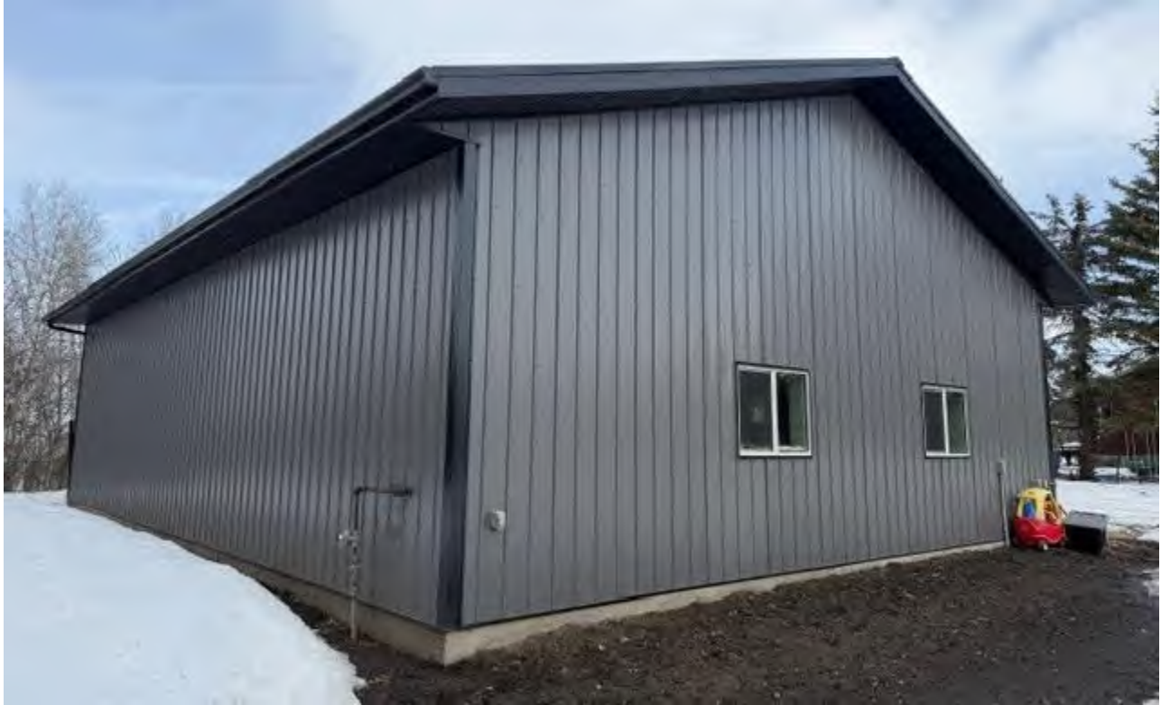
Rear/side of detached garage/shop – notice gas connection.
