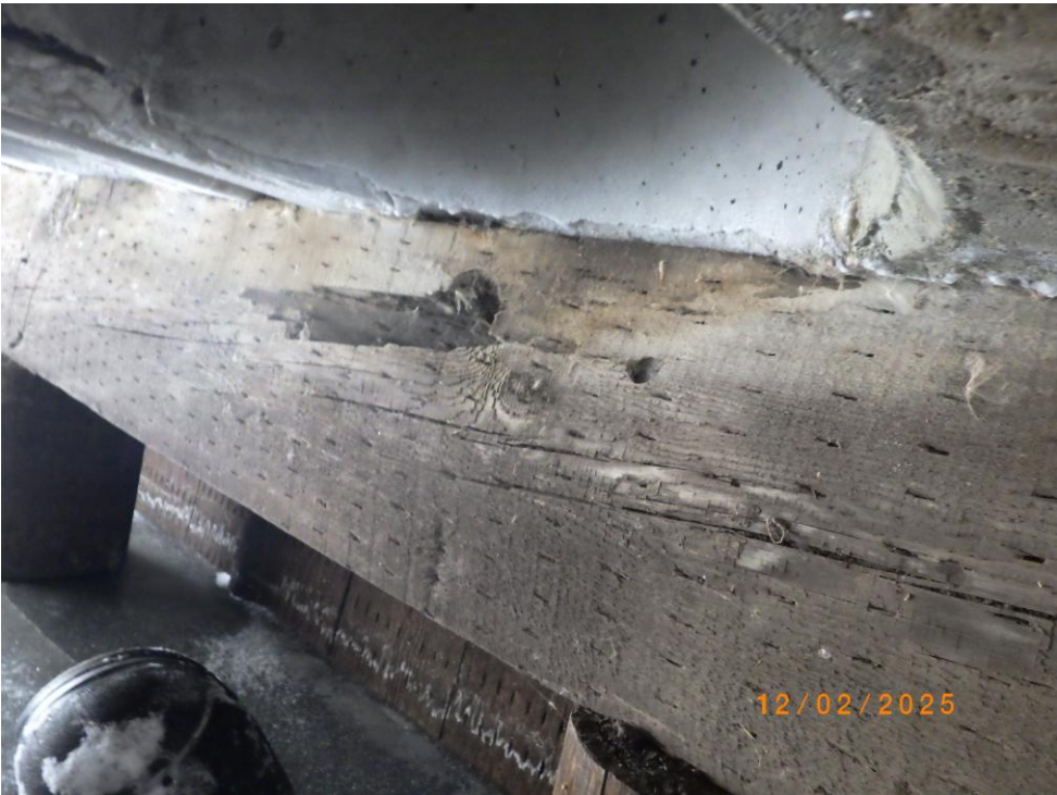
Another tieback bolt pulled into crushing cap
